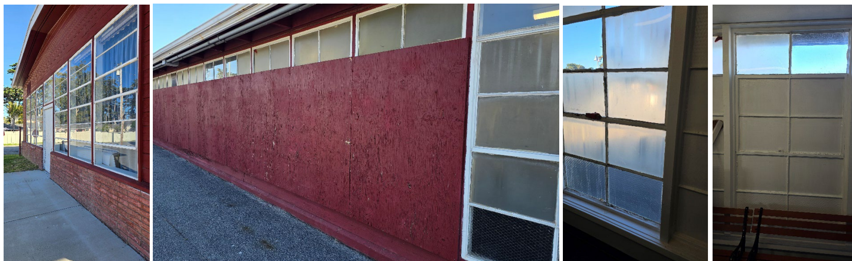
Pacific Grove Adult School Windows in Poor Condition
